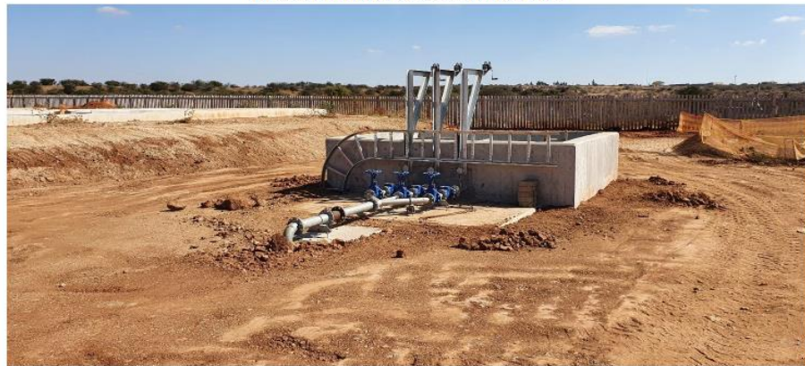
Supernatant pump sump.
