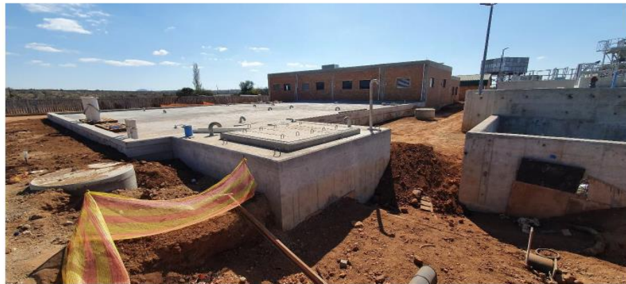
Reservoir inlet chamber and reservoir.
