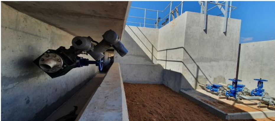
Clarifiers and heavy / light solid sumps.
