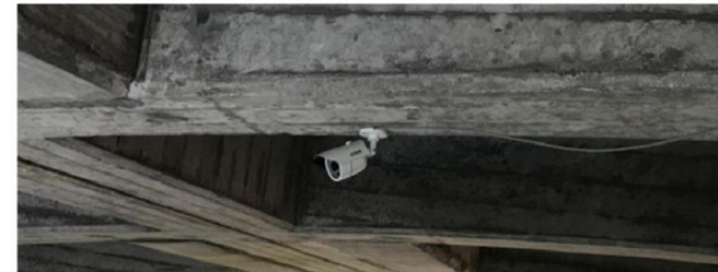
Wireless solar powered cameras used on California and Pennsylvania scour critical bridges.
